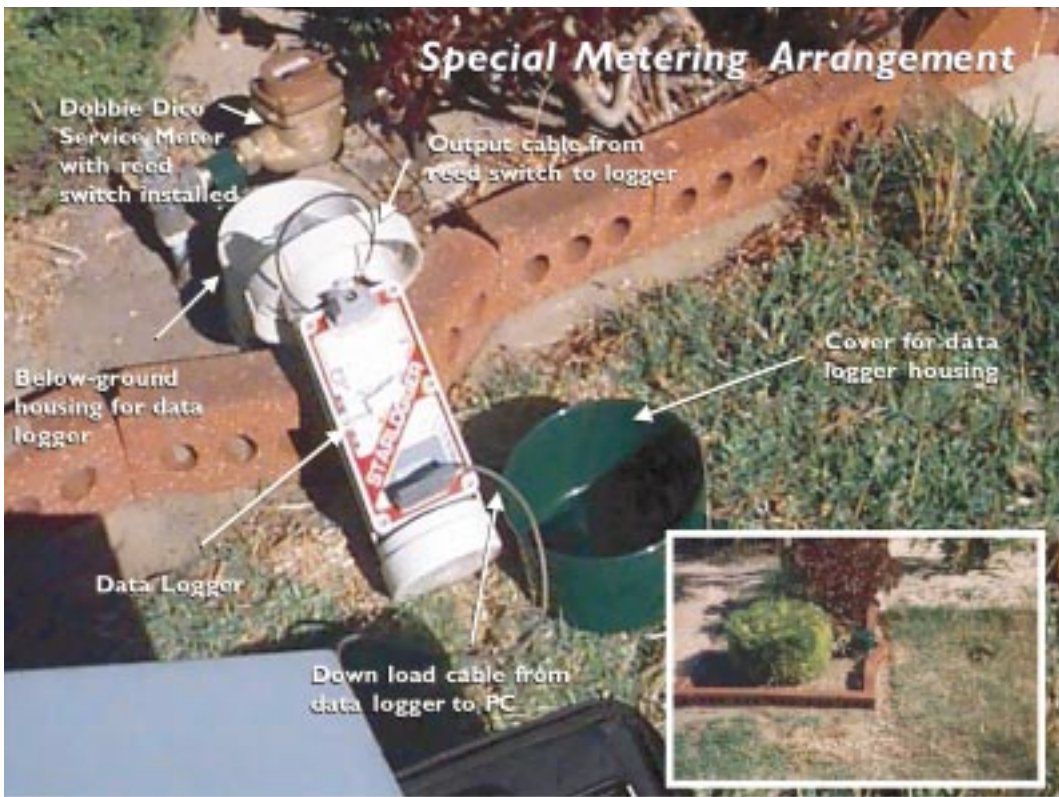
Figure 1.3 ~ 'Smart' Meter Arrangement
