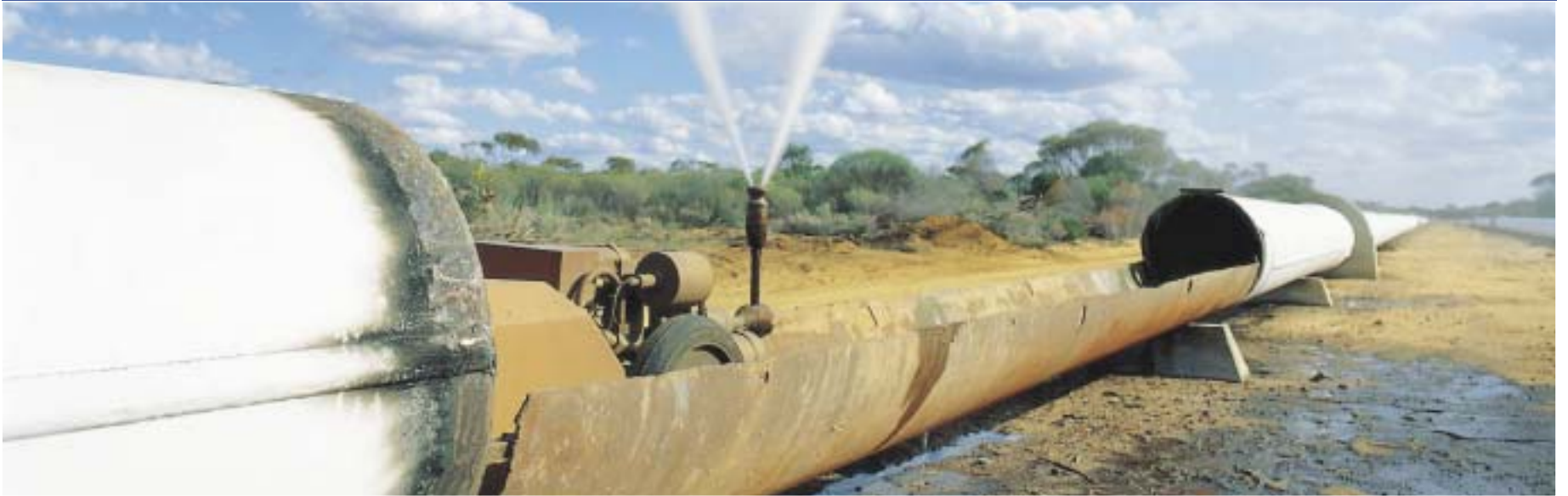
World-class water supply scheme - Since 1903, the historic Goldfields pipeline has been continuously upgraded to meet demand.
