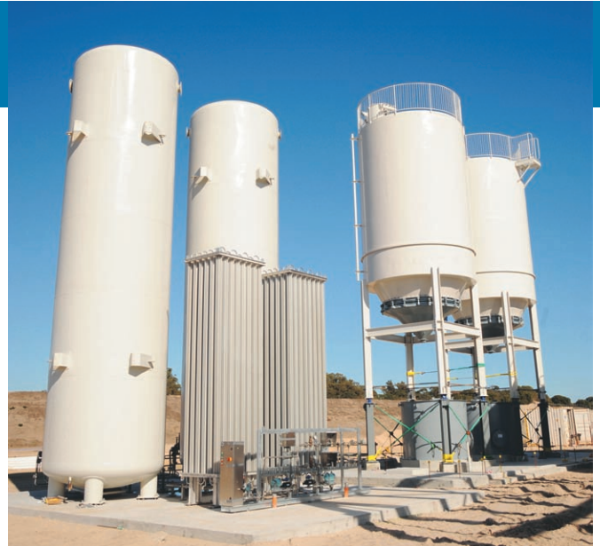
Potabilisation Area including lime and CO 2 storage.
