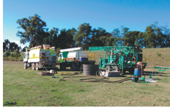
First action on site – a drilling rig being prepared to enable initial soil testing to begin
