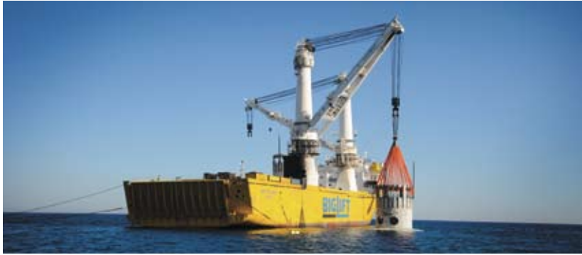
The first 400 tonne seawater intake tower being lowered into the waters off Binningup.
