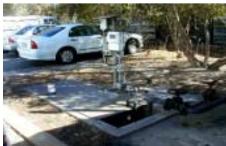
A typical Industrial Waste sampling and monitoring facility
