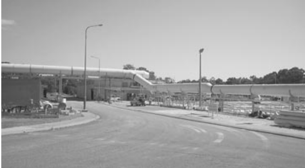
New ducting to take odorous air for treatment.
