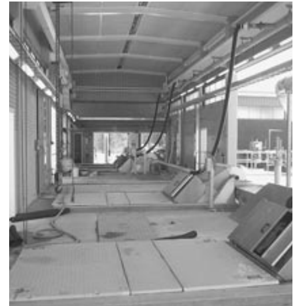
New covered screens to filter wastewater entering the plant.
