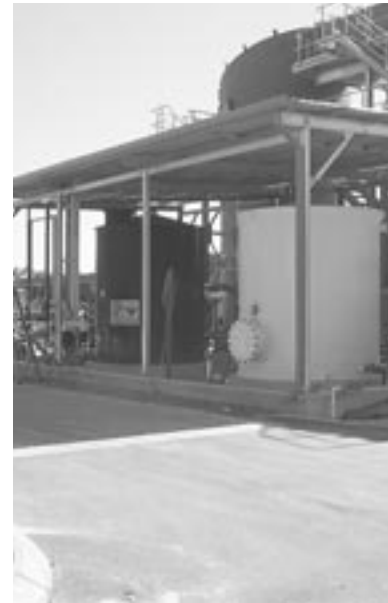
New chemical dosing plant for the scrubbers.
