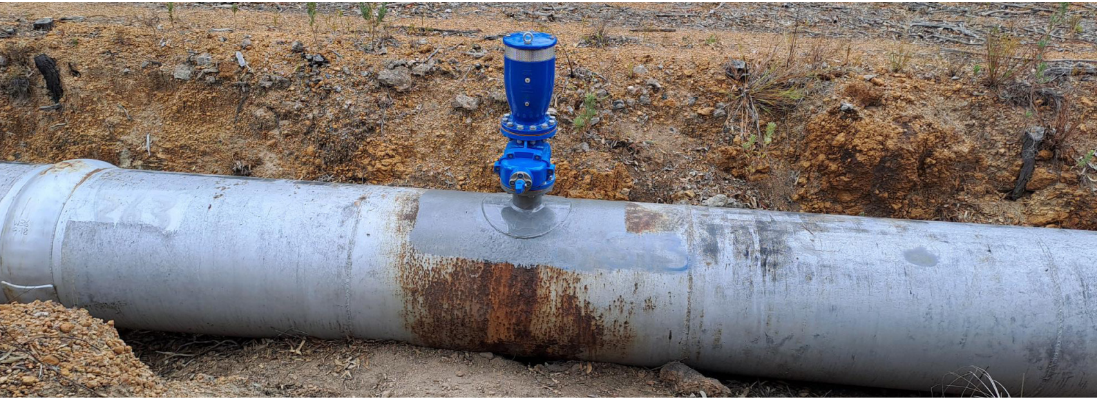
Image 56: GWSS, new air valve at Bakers Hill
