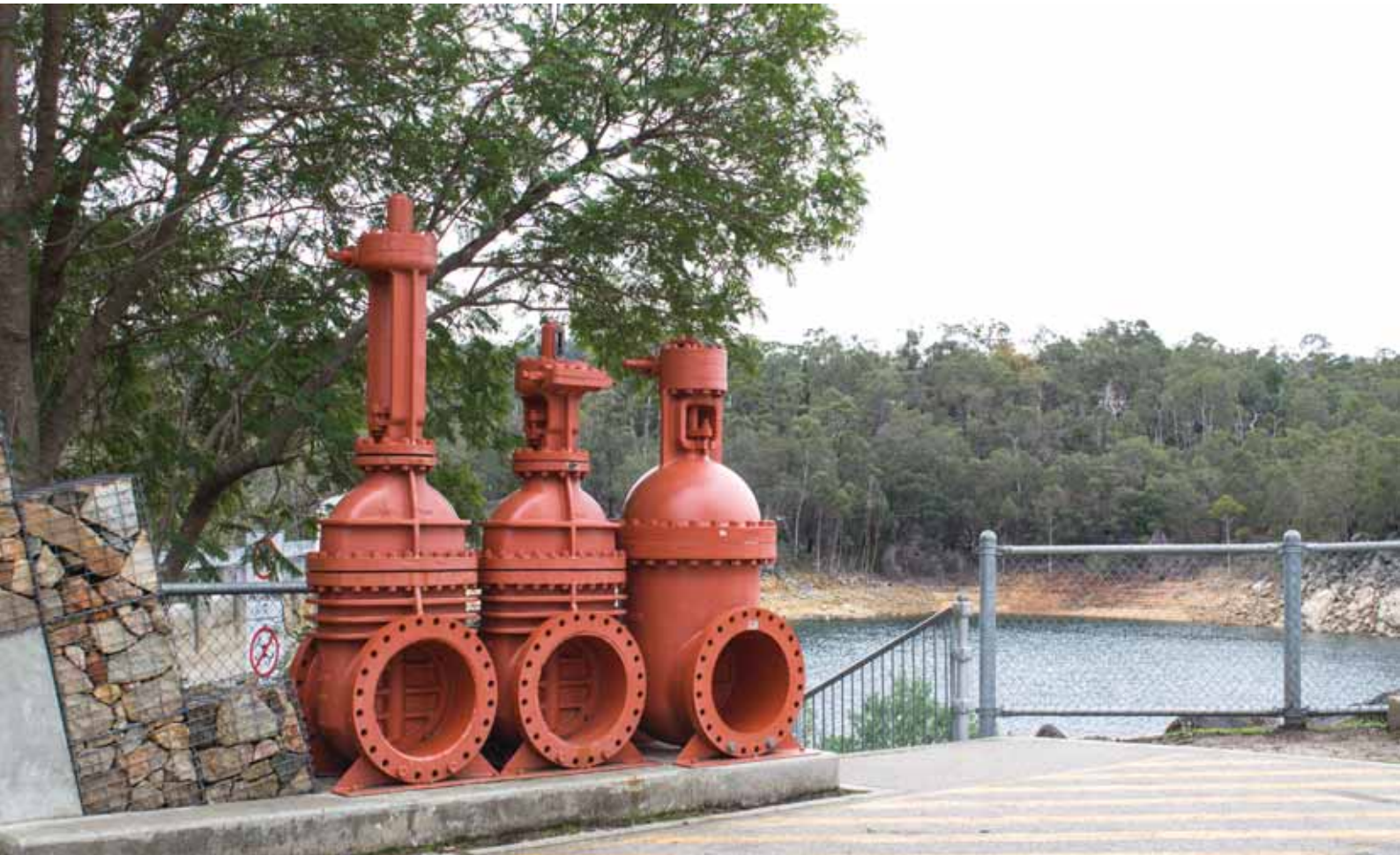
Image 57: Image of GWSS pipe valve interpretation
