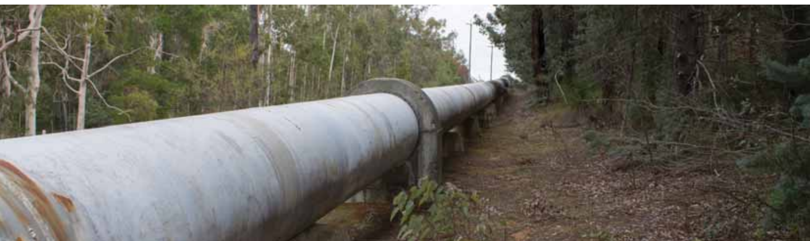
Image 45: GWSS Main Conduit at Fred Jacoby Park
