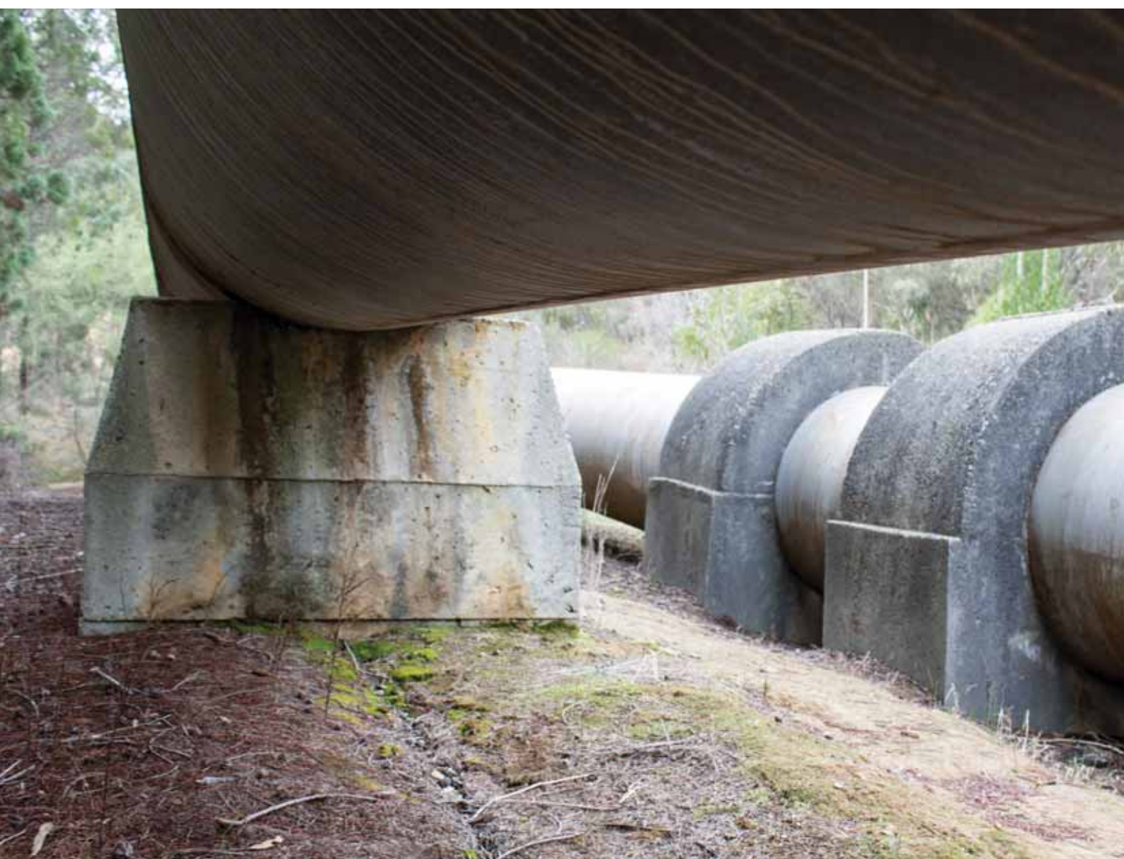
Image 7: Anchor blocks insitu at Fred Jacoby Park
