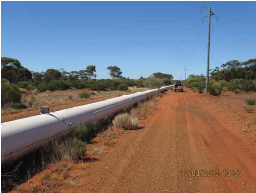
Photograph 05 Locking bar pipe near Coolgardie Water Corporation, March 2015
