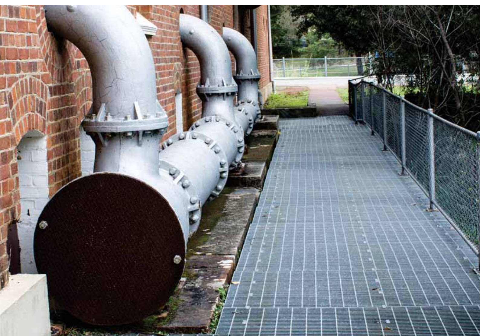
Image 17: GWSS main conduit at Pump Station no. 1
