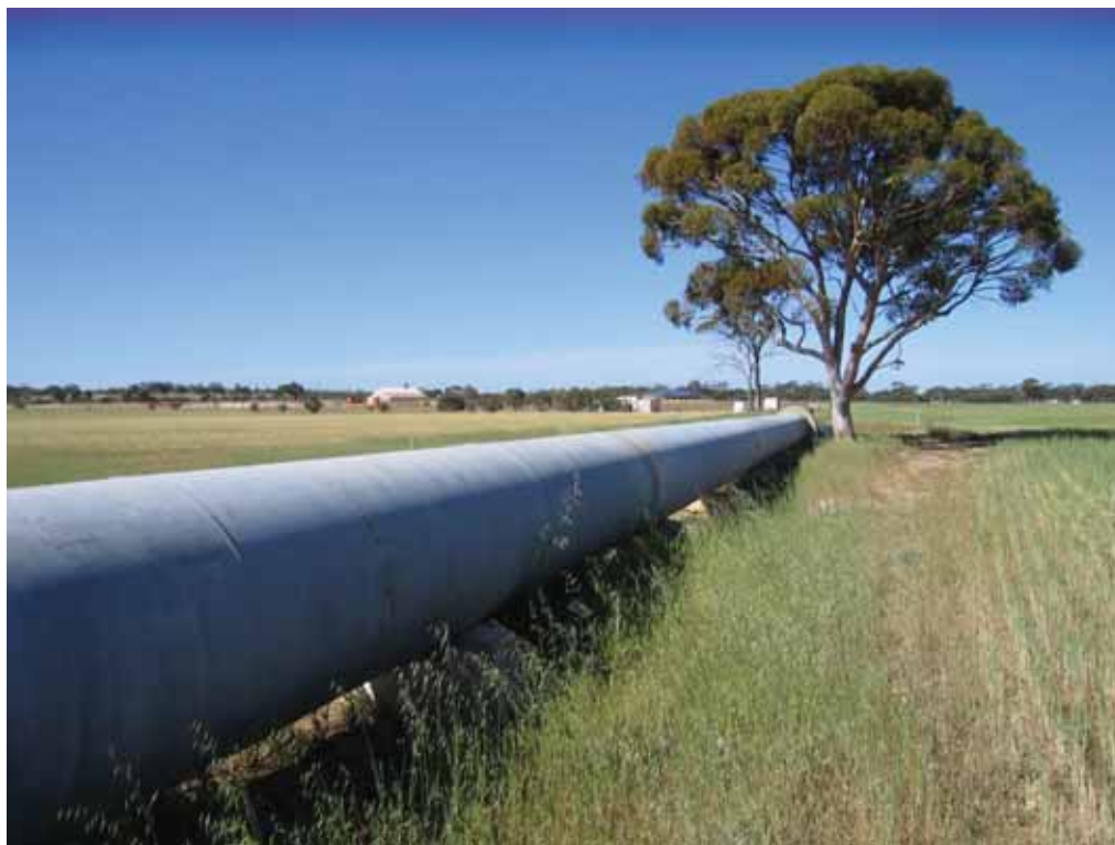
Photograph 07 MSCL pipe Water Corporation
