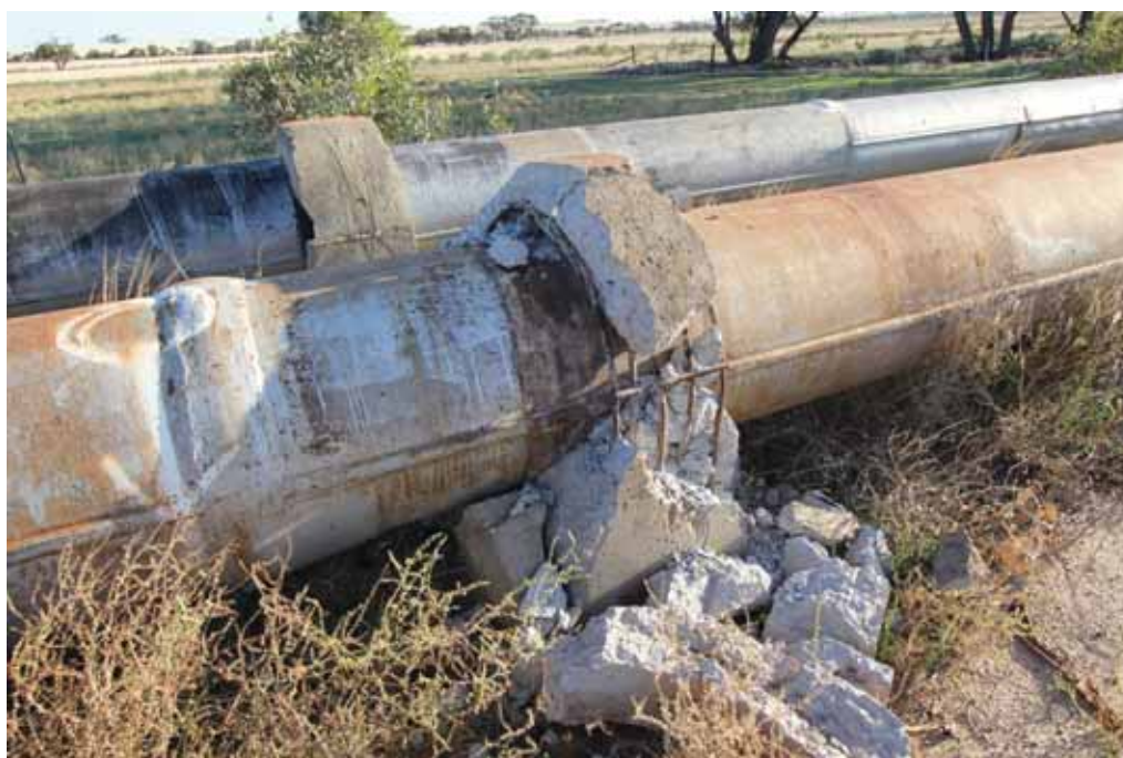
Photograph 02 Deteriorated concrete anchor near Meckering Griffiths Architects, April 2016
