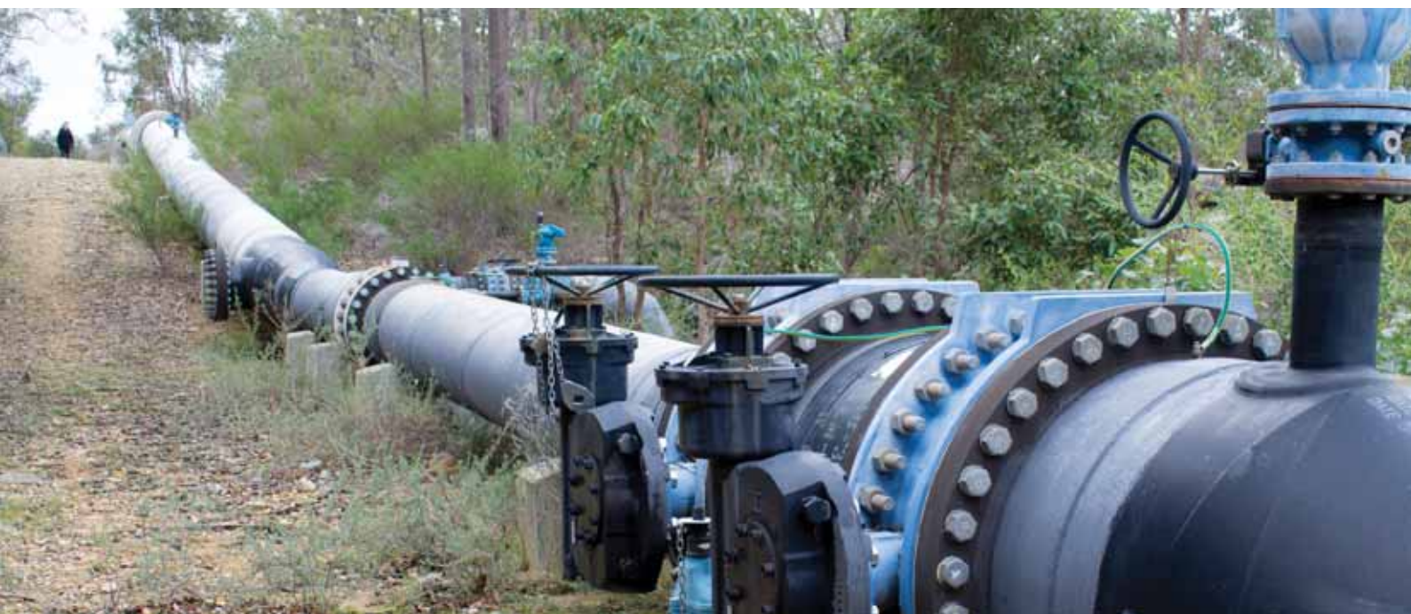
Image 5: MSCL pipe with a spiral weld near Mundaring Weir
