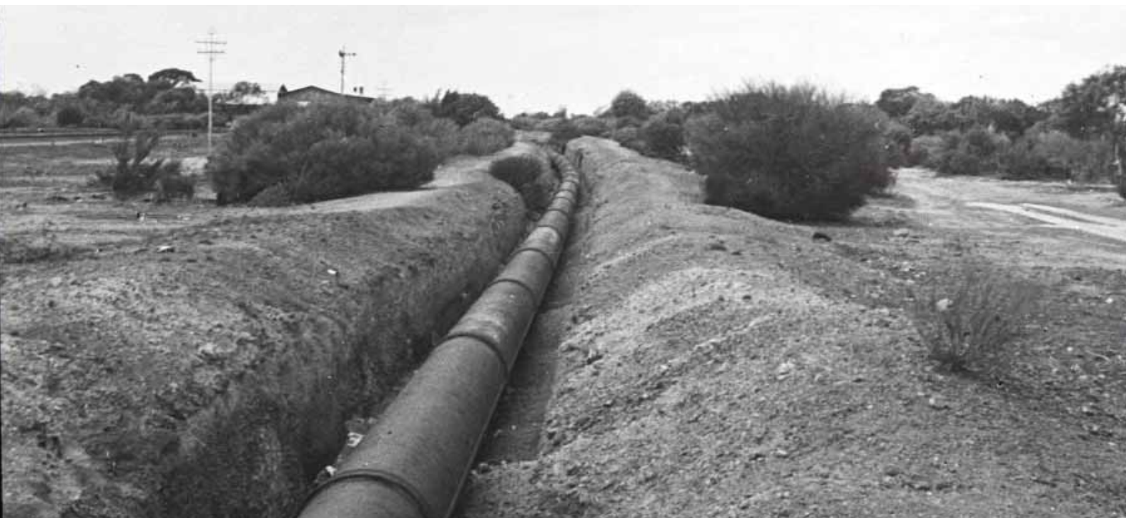
Image 31: The Goldfields Water Supply Scheme pipeline
