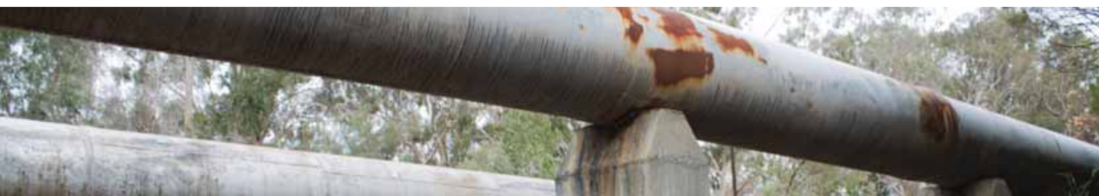
Image 46: Elevated Main Conduit in Fred Jacoby Park
