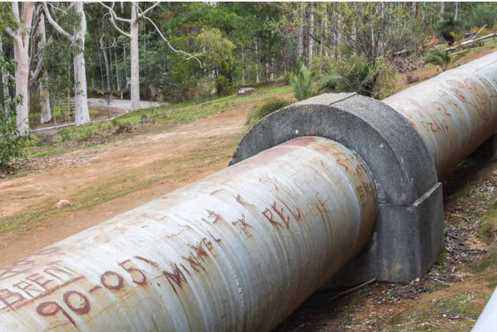
Image 54: Inscriptions on the pipe at Fred Jacoby Park
