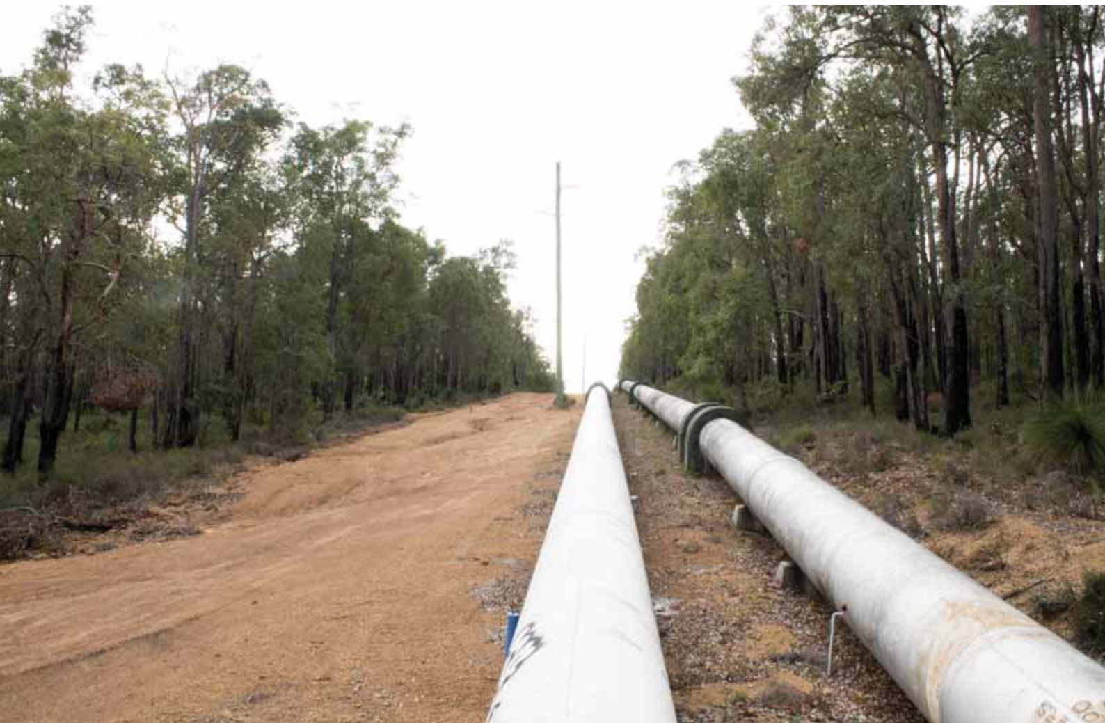
Image 42: GWSS Main Conduit at Mundaring
