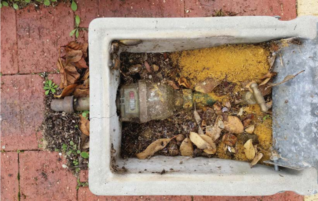
This box is not an approved box and it doesn't allow us to replace the meter.
