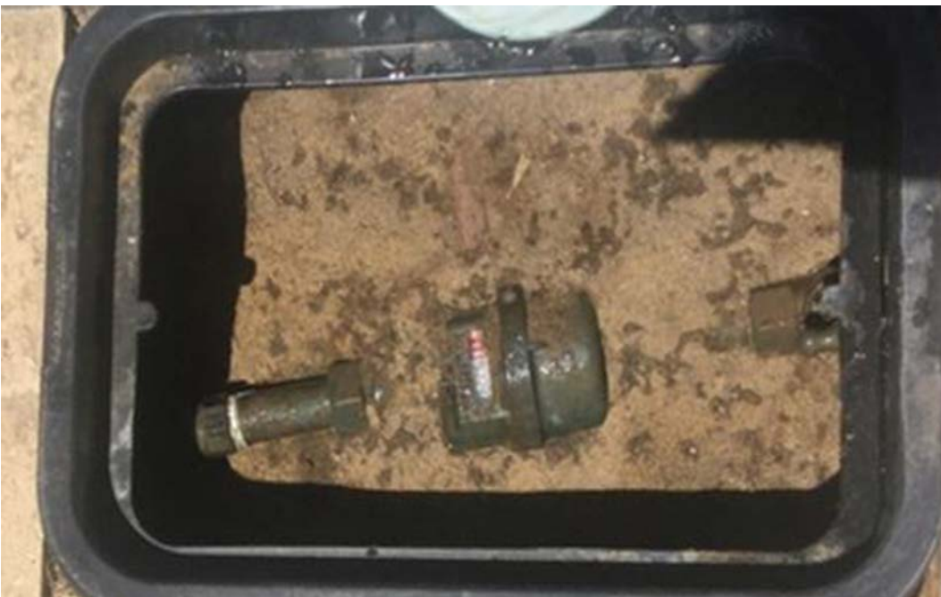
This box is not an approved box and has resulted in a build up of soil covering the meter.
